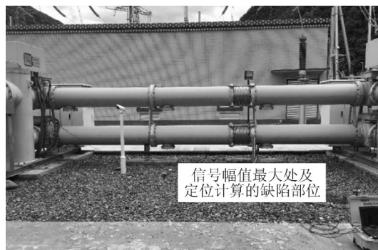
图9 110 kV 缺陷盆式绝缘子特高频测点和放电源位置 Fig. 9 UHF measuring points and defect position of 110 kV pot insulator with surface discharge
